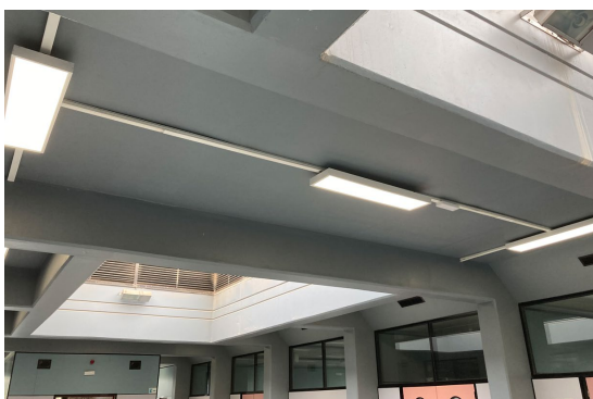
Luminarias Led en hall
